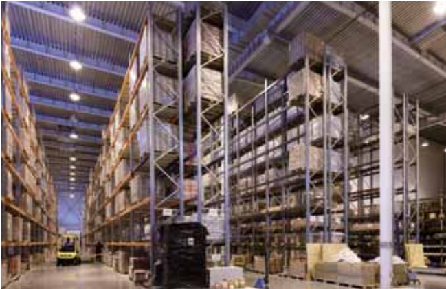
High bay lighting
